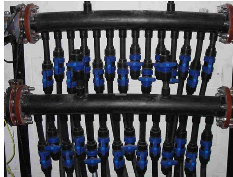
Port Hawkesbury geothermal system
